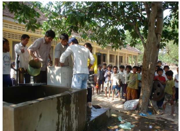
Students watch our crew installing a bio-sand filter at the Lboeuk primary
